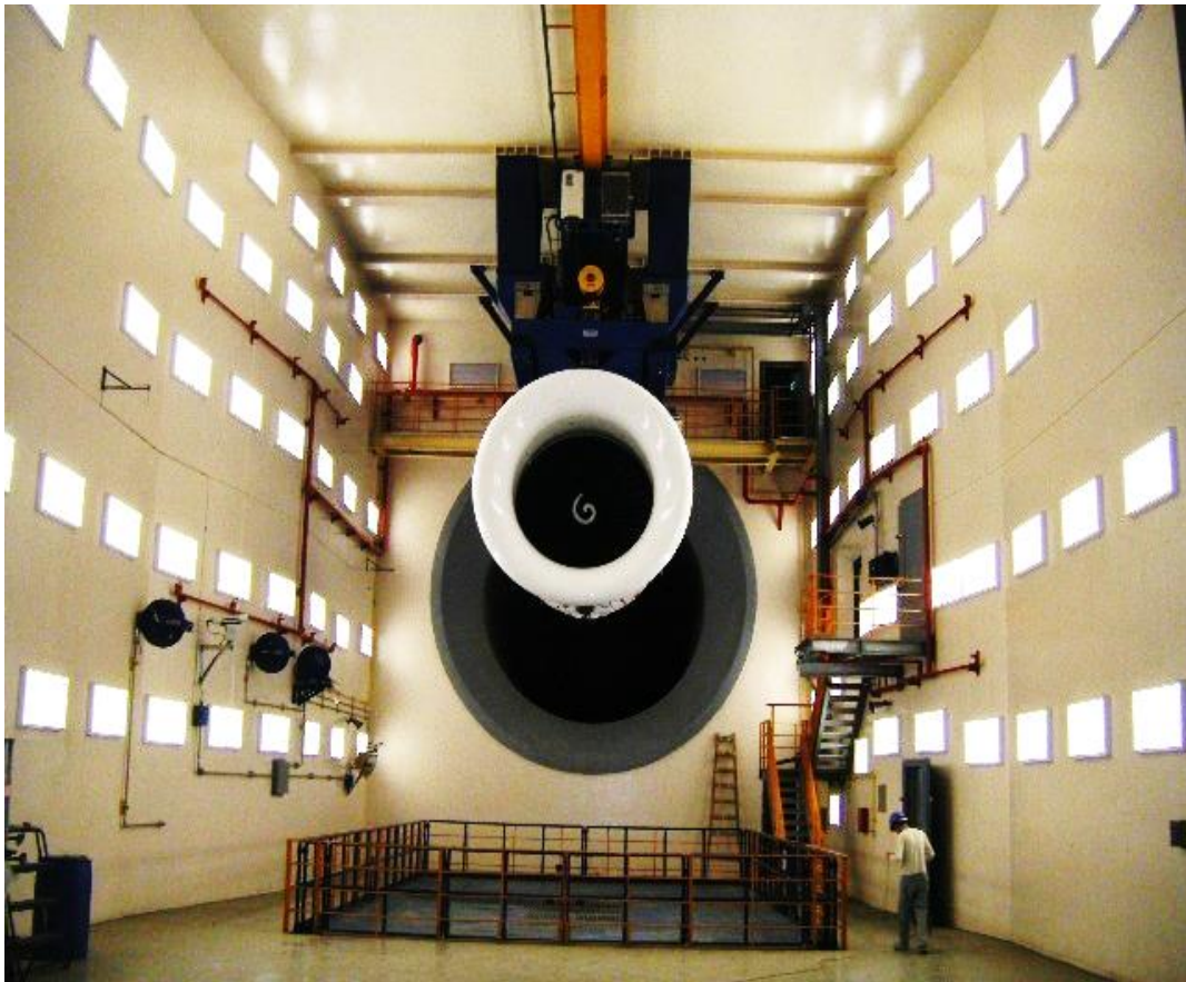
Engine Test Cell
